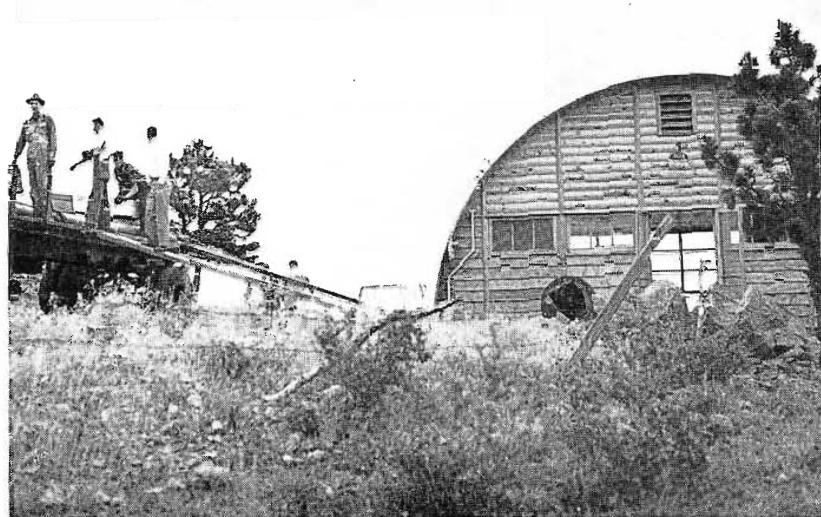
FIG. 10. Rear view of transmitter building. Antenna was installed in lower right foreground.
