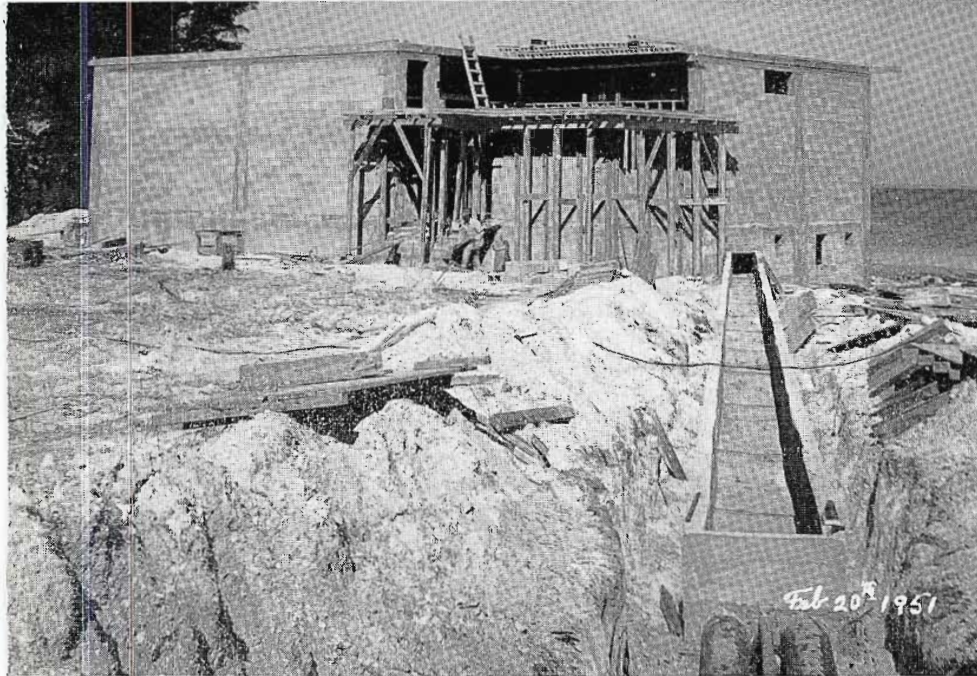
FIG. 10. Construction of WSUN transmitter building, from roadway between towers. Note pre-fabricated hollow concrete roof-joists, and, in foreground, cast-iron conduit and concrete trough for southeast tower lines leading to basement.
