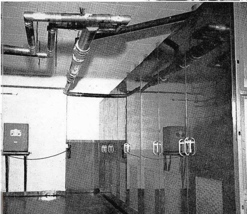
FIG. 10. Shown here is the 25-KW Diplexer completely installed and ready for high power operation. Note that it was possible to feed the TT-5A driver into the antenna system by simply changing two co-axial runs.
